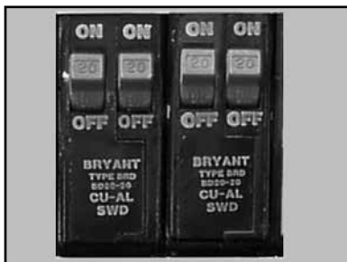
(D) Verify the circuit breaker is at least 20 amps – if not, move to 20 amp circuit.
