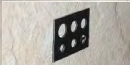
Stick the guide pad onto the clean, dry tile. The corresponding size hole to the diamond crown should be selected in line with the mark
