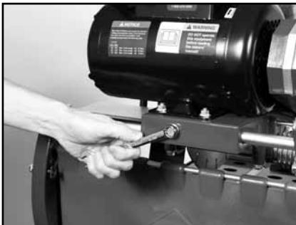
(D) Verify the Motor Adjustment Strap is tight.
