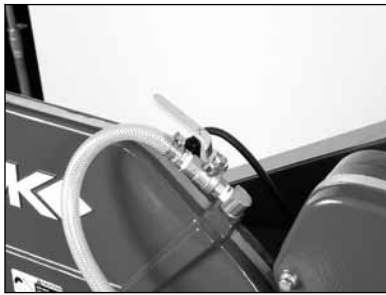
(A) Check Cooling Flow Control Valve is open.
