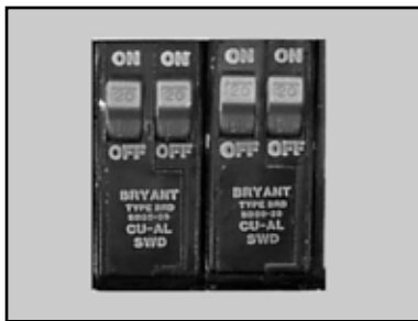
(E) Verify circuit breaker not tripped if tripped, reset once
