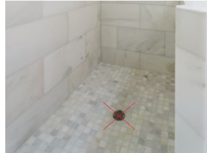
Standard Drain in Center
